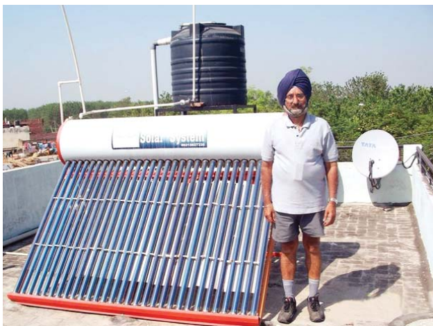
Grewal makes full use of technology. This solar panel gives them enough warm water, and therefore power cuts do not affect them. The house is built such that in summer it remains cool all through. Even though air conditioners are installed in every room, and they have full power backup, he actually does not need even a fan for most of the year. The cool air under the trees is exhilarating!
